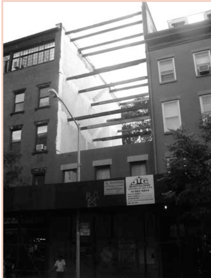
178 Bleecker Street, an 1861 house in the South Village, was demolished over GVSHP's objections and without intervention by the city.
